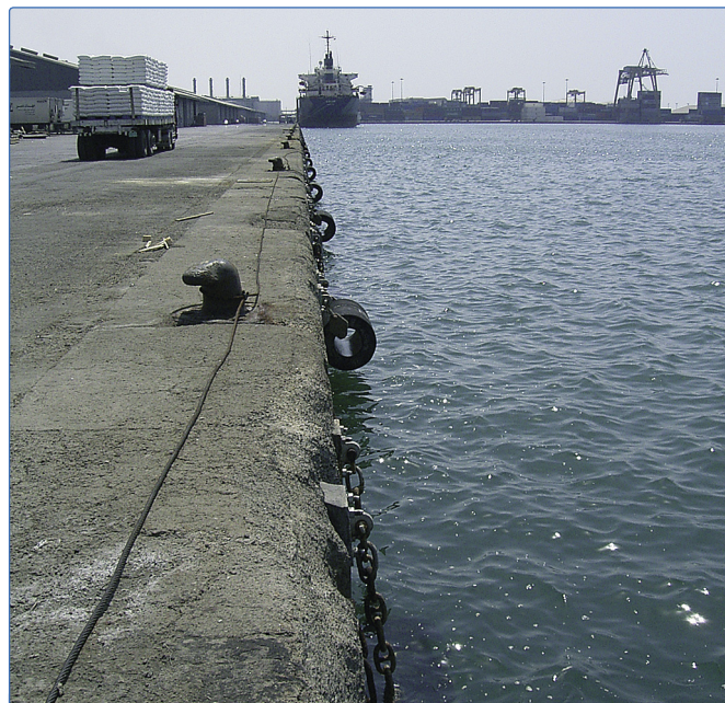
Corrosion of chains and accessories are a principle cause of early fender failure.
